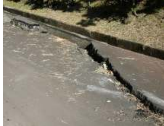
Slumping on a road: this road is sliding downhill slowly.
