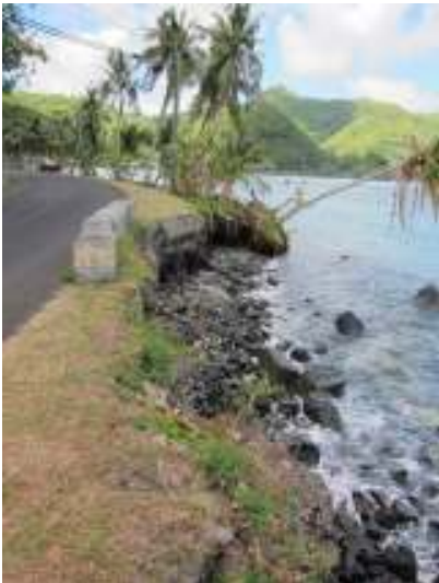
Shoreline erosion at Faga'itua
